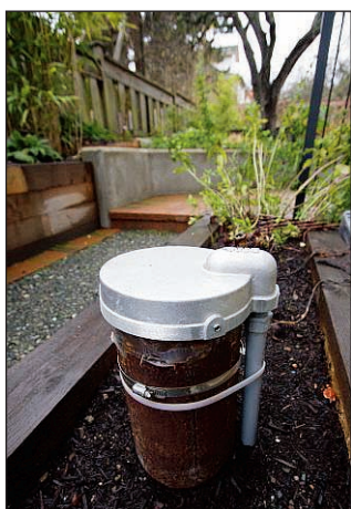
DARREN STONE, TC A geothermal wellhead to bring heat from the Earth.
